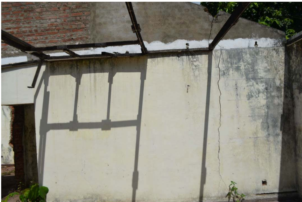
Figure 11: Cracks in Bungalow building (location: near top of slope, GPS-4 position in Fig. 9)
