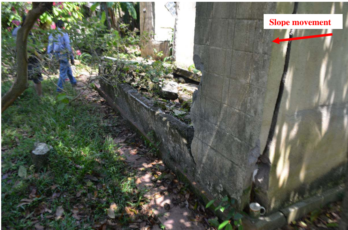
Figure 7: Damaged houses near the toe of slope.
