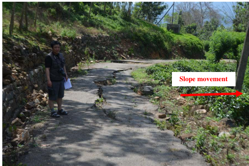
Figure 13: Damage to road along location GPS-2.
