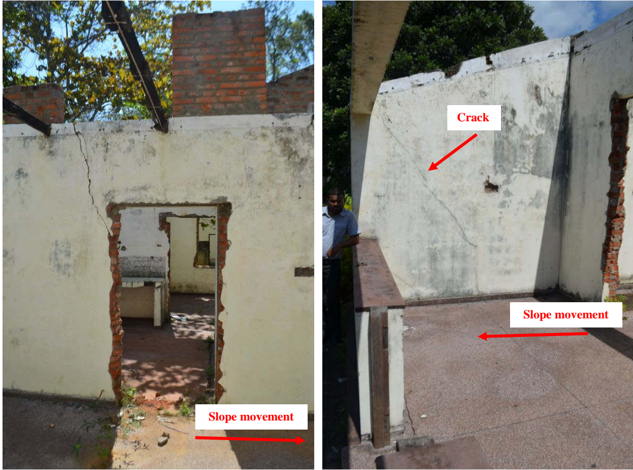
Figure 12: Cracks in Bungalow building (location: near top of slope, GPS-4 position in Fig. 9)
