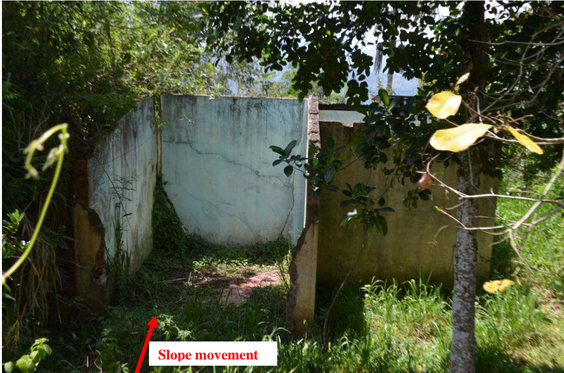
Figure 8: Damaged houses near the toe of slope.
