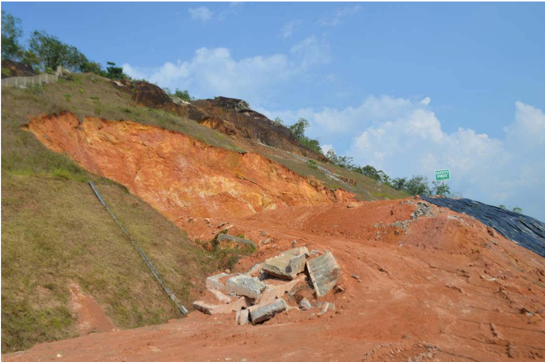
Figure 16: Overview of Dodangoda landslide site.
